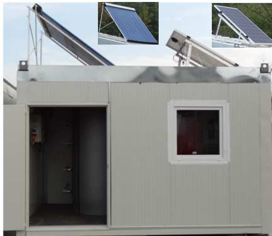
Fig. 4 - Heating plant by capitalizing the energetic plant Miscanthus IIVM
